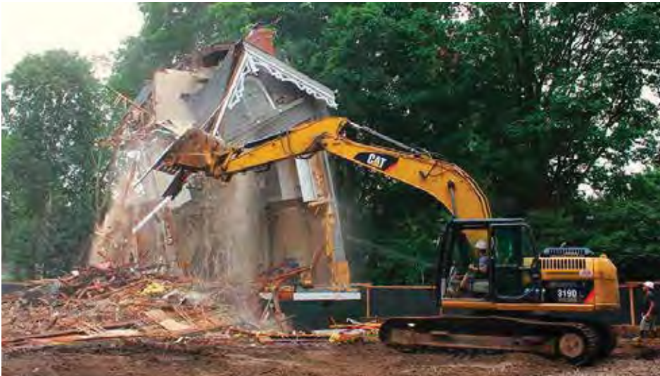
The A.T. Stewart-era house at 104 Sixth Street, Garden City, was demolished on August 1, 2016. (Courtesy Garden City News Online)
